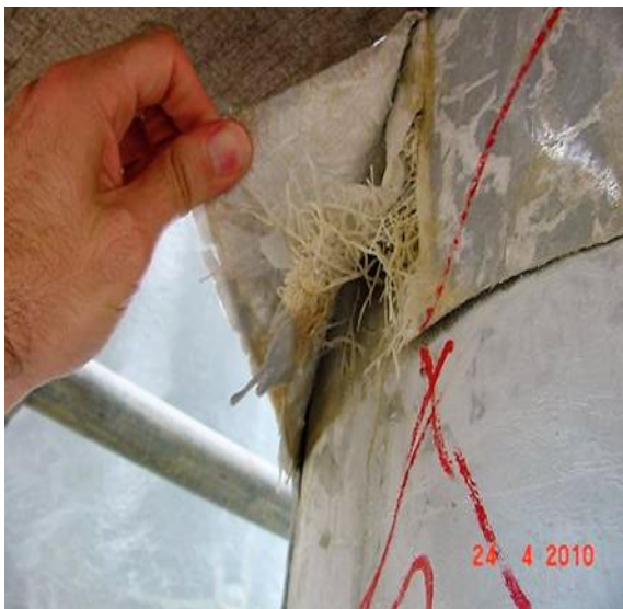
Poor adhesion of wet-applied GRP. Removal of this piece may result in damage to the underlying insulation. A new piece of uncured GRP is also required.
